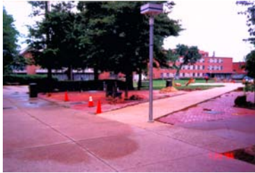
Existing student plaza in disrepair
